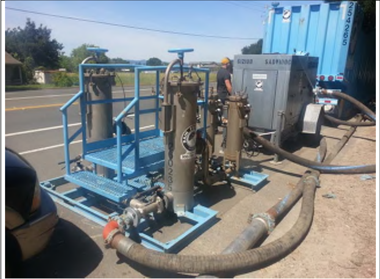
Bag filters used for sediment removal prior to discharge of water to sanitary sewer.
